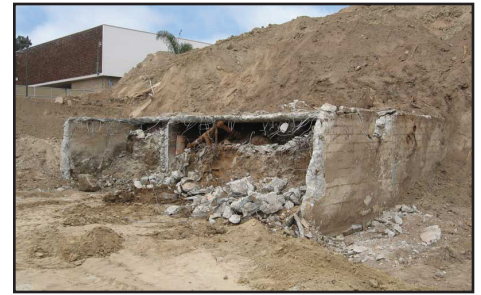
Part of the fresh-water cistern uncovered during recent grading on campus. An old road was also uncovered and had to be removed.
